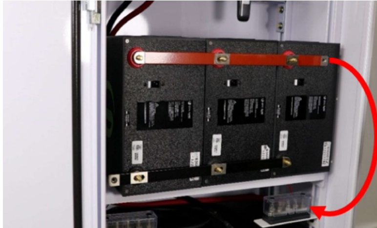
Figure 8.0 - PHI Battery Wiring Using Interconnecting Busbars
